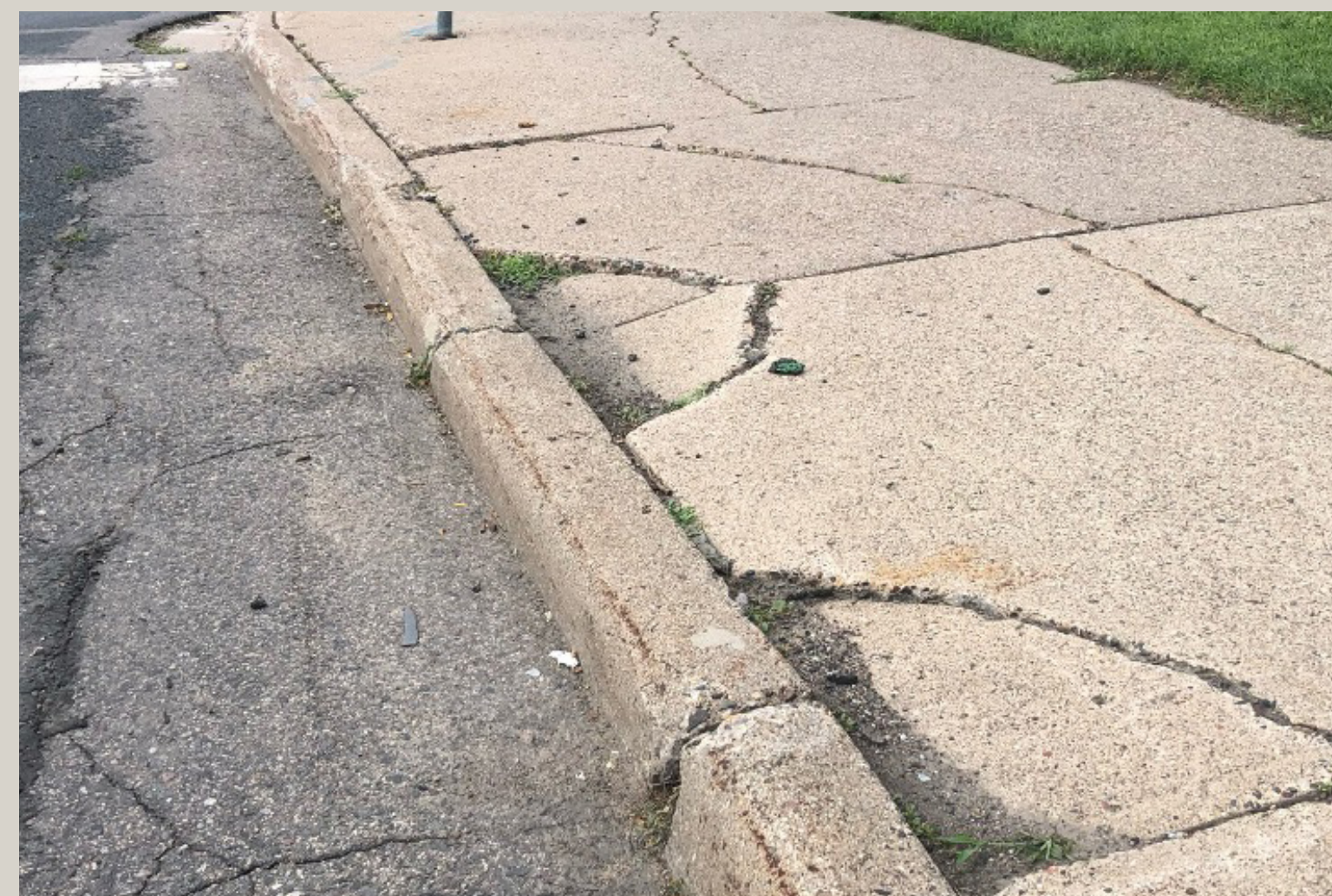
Broken, uneven sidewalks
