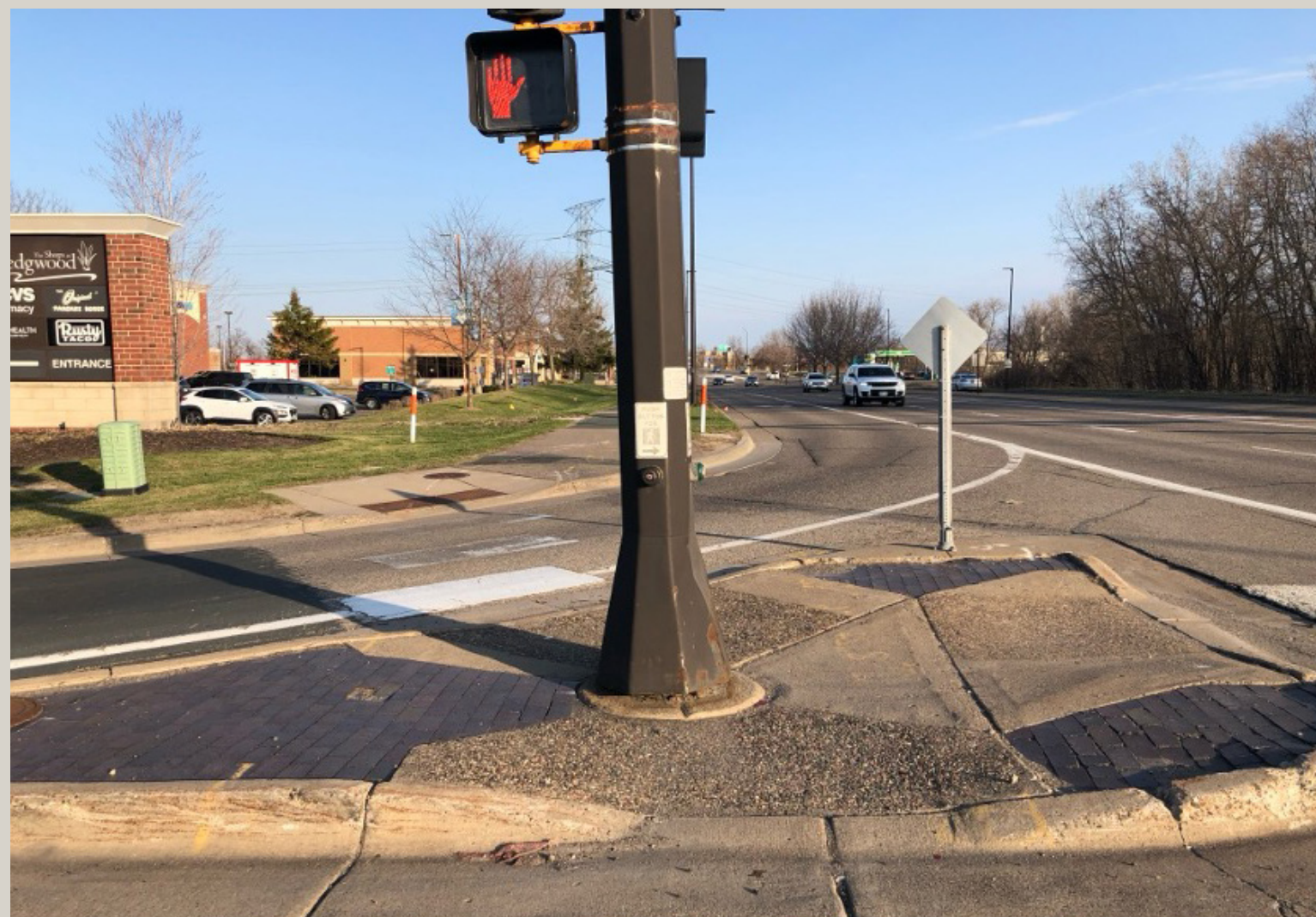
Obstructions in the middle of pathways
