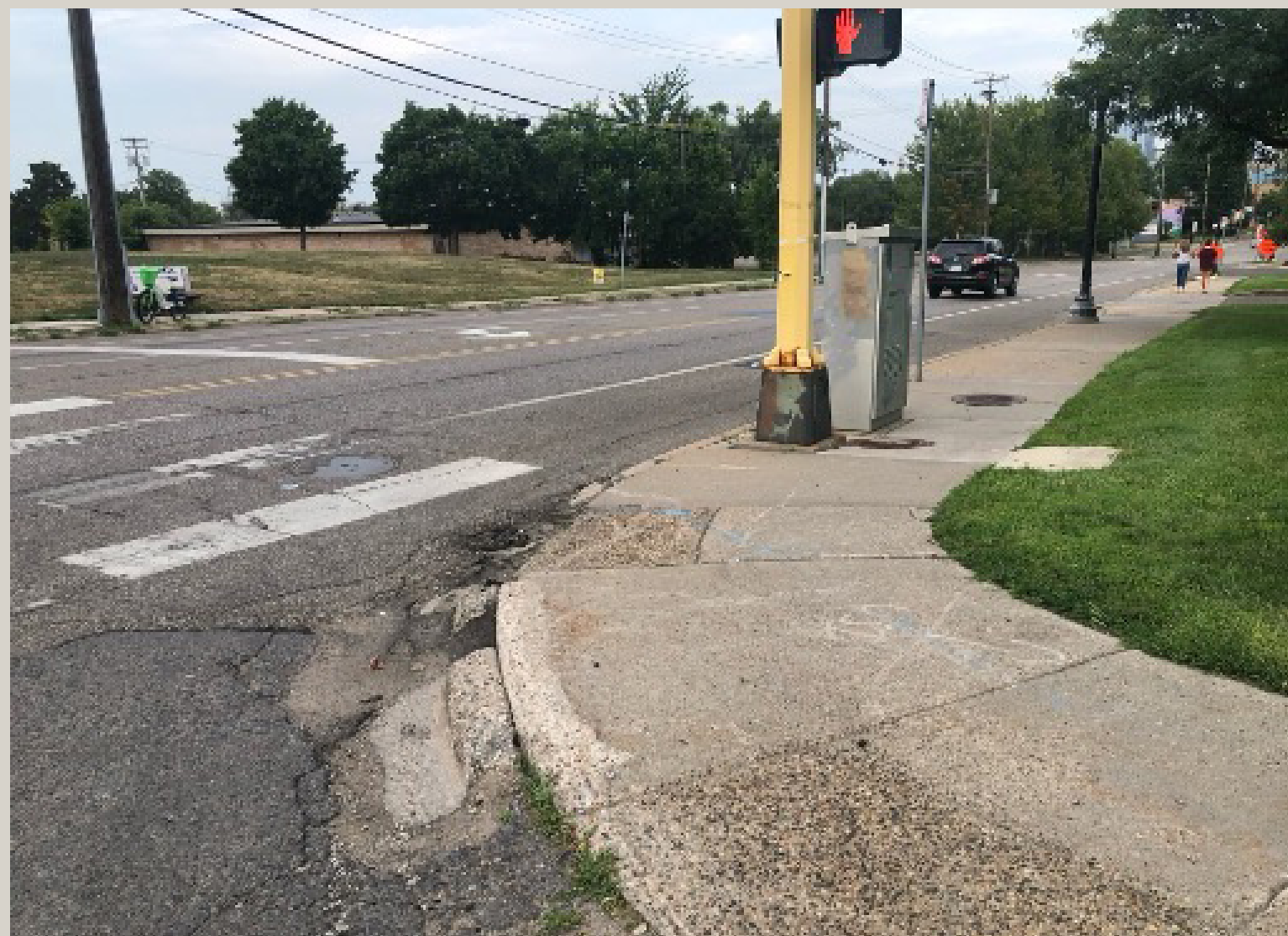
Narrow, uneven ramps
